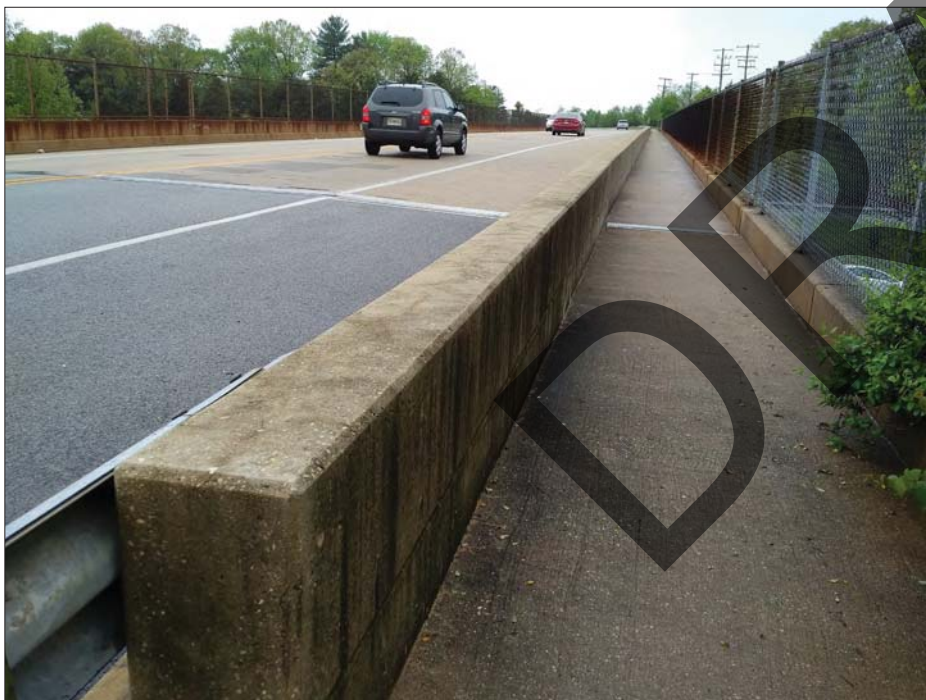
This buffered sidewalk along Gorman Rd across I-95 is an example of acceptable pedestrian accommodation across a limited-access highway.
